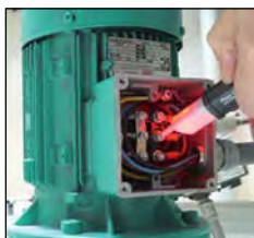
Incorrect phase sequence
